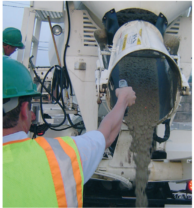
Estimating the temperature of fresh concrete as it enters the chute. This temperature is approximately the same as the required ASTM temperature test.
