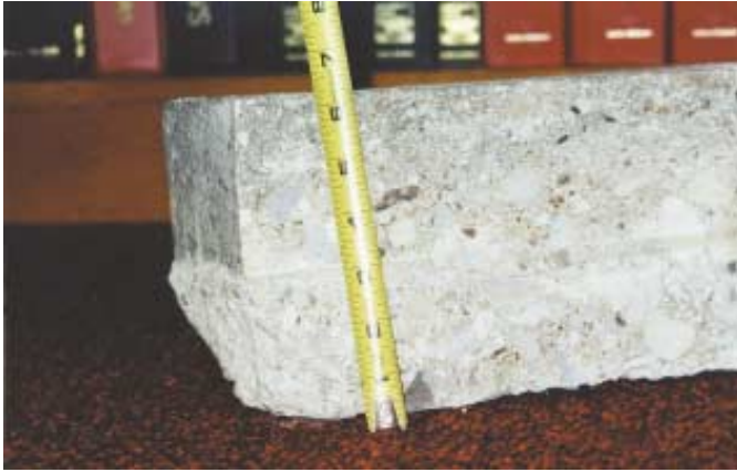
A piece from the Bellefontaine concrete pavement that shows the full depth (note the two layers of pavement)
